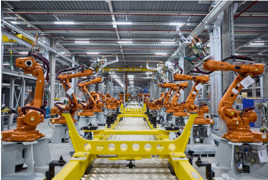
© BMW Group System installation in the new body shop, BMW Group Plant Munich (02/2025).
