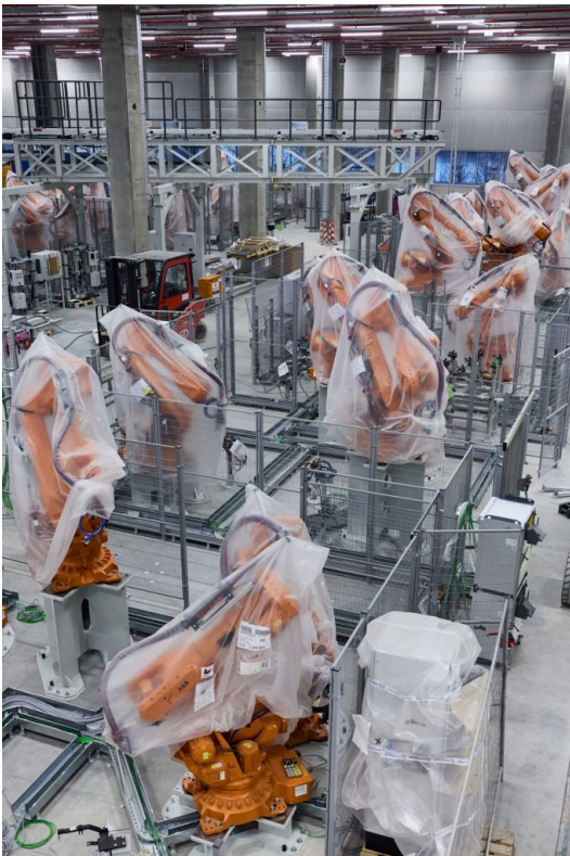
© BMW Group System installation in the new body shop, BMW Group Plant Munich (02/2025).
